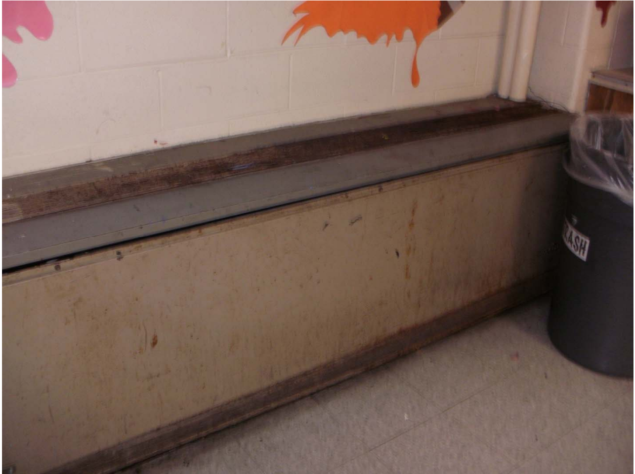
Photo No. 4 – Typical Classroom Unit Ventilator.
