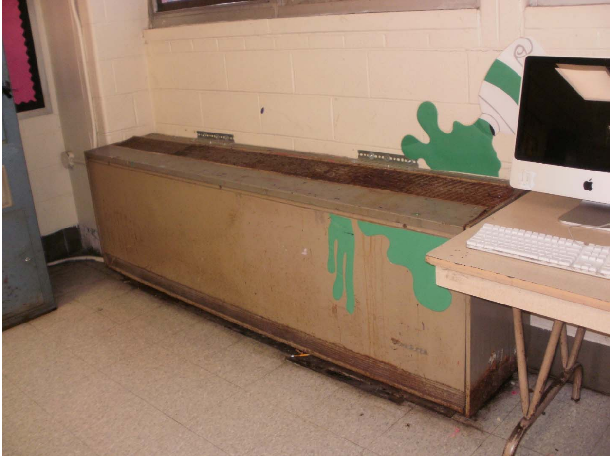
Photo No. 3 - Typical Classroom Unit Ventilator.
