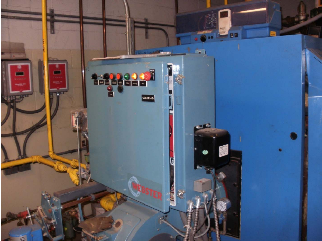
Photo #1 – New Webster Boiler No.3 installed @ 2010 Located in the Boiler Room.
