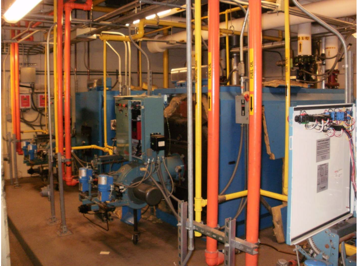
Photo No. 6 – The 3 Boilers in the Basement Boiler Room
