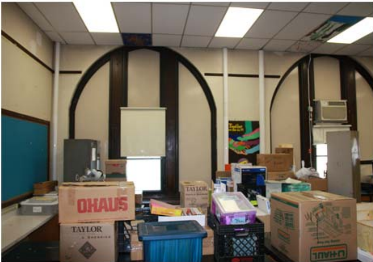
Typical window at Lab 406. Refer to Drawing A1.01 for quantity. Each window is approximately 48" wide x 80" tall.
