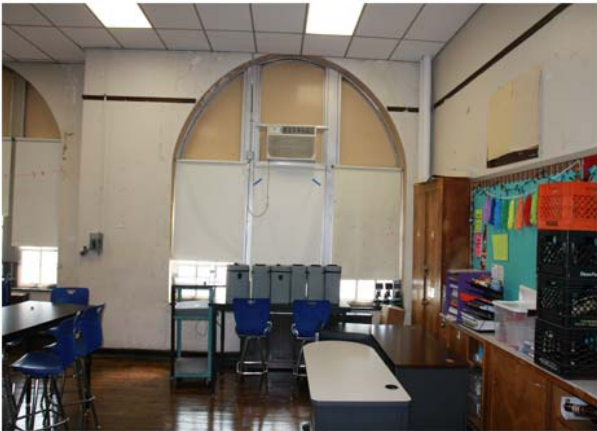
Typical window at Lab 404 and Prep Room 403A. Refer to Drawing A1.01 for quantity. Each window is approximately 36" wide x 90" tall.
